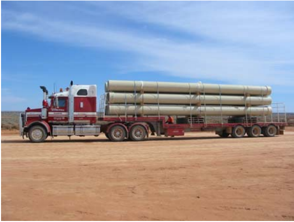
Figure 3: A batch of 12 metre length GRP pipes being delivered to the J-A site. Longer pipes require fewer joints per unit length, simplifying the installation process.
